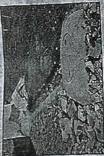
MAKING IT LEGAL: A sewage connection on the encroached land
